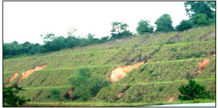
Figure 7.6. Localised slip failures and erosions on slopes.
