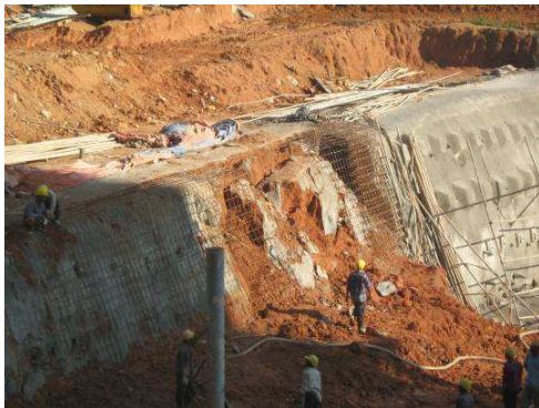
Figure 2 Localised surface slips occurred during soil nailing work
