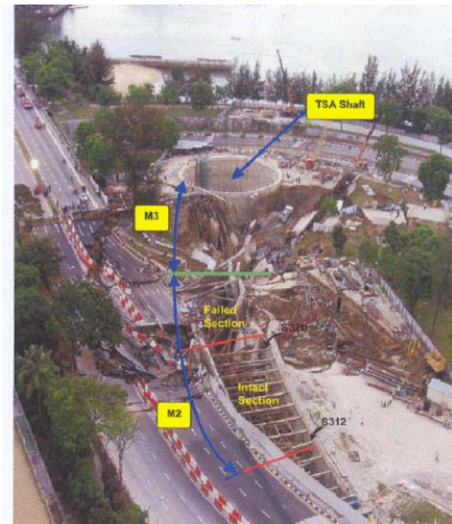
Fig. 3 Nicoll Highway collapse (COI, 2005).
