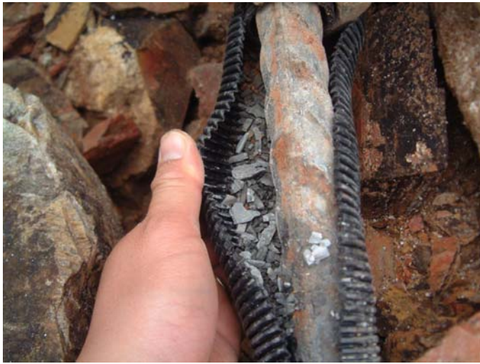
Fig. 8 Grout cracked and peeled off from nail – ineffective corrosion protection.
