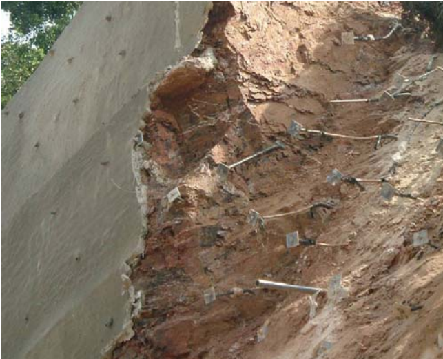
Fig. 10 Example of face failure (side view).
