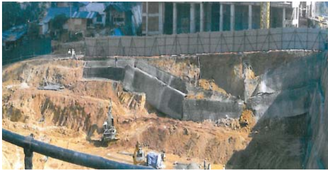
Fig. 16 Failed soil nail slope (Note: Some backfilling works already carried out to stabilize the slope).
