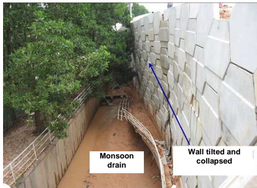
Figure 4 Side view of the collapsed combined wall
