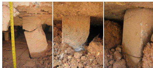
Figure 12 Settlement of piling platform and flexural damage of embankment foundation piles
