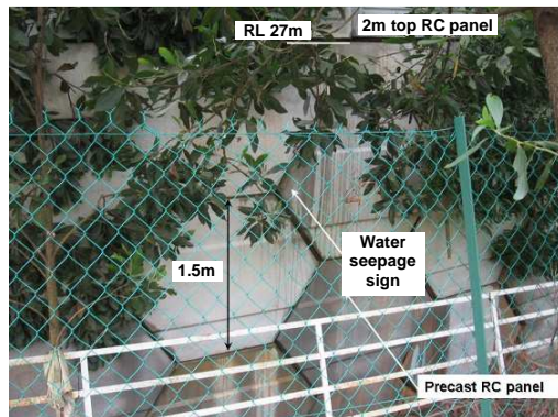
Figure 5 Observed watermarks on wet wall panels
