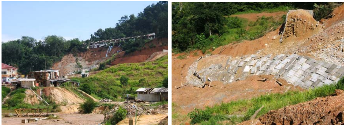
Collapse of Reinforced Soil Wall at Kampung Pasir on 31 May 2006
