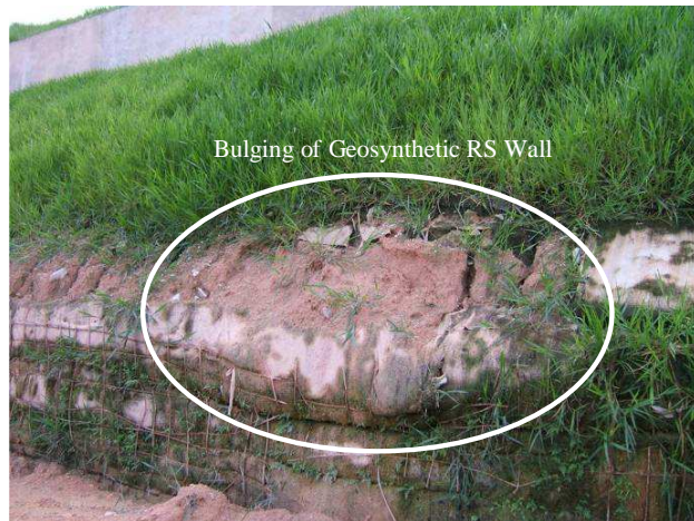
Figure 8 Bulging of Geosynthetic RS wall
