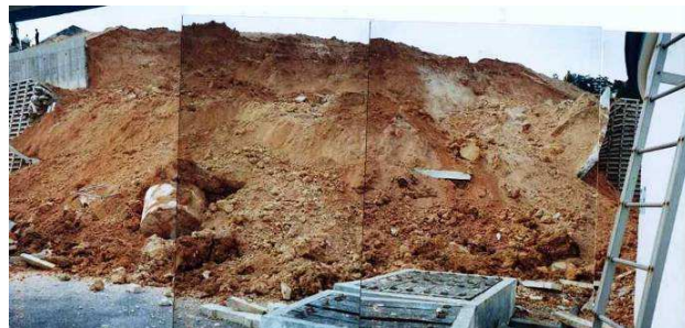
Figure 1 Collapsed Crib Wall and Piled RC Wall
